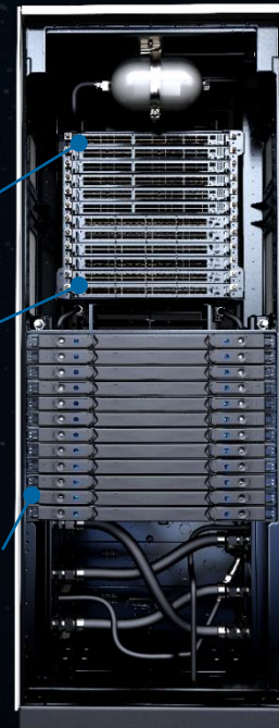
42U Cabinet Rear View
