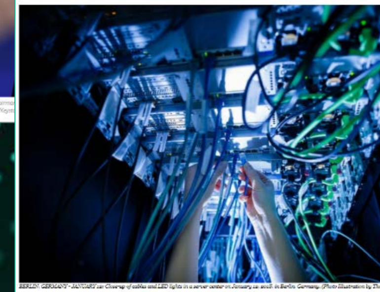
BERLIN: GEORGIY ANTONOV in Closing of cables and LED light in a server center in January 2018 in Berlin, Germany. (Photo illustration by The
