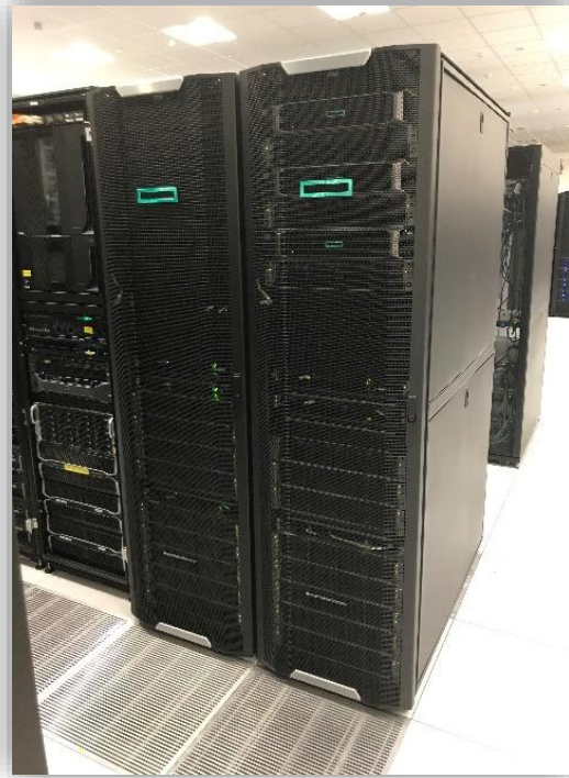
Fulhame Catalyst system at EPCC
