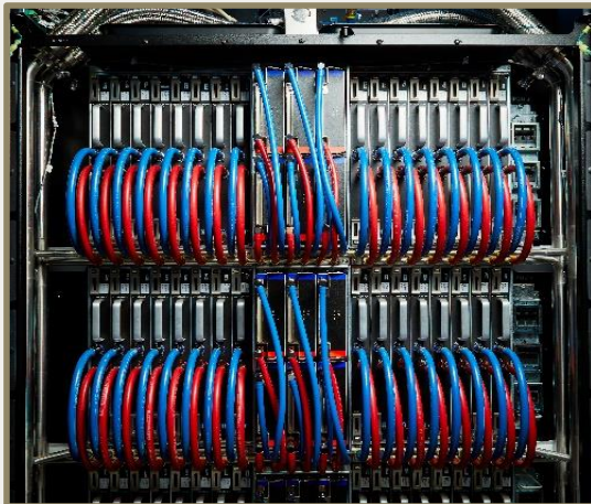
Direct liquid cooling
